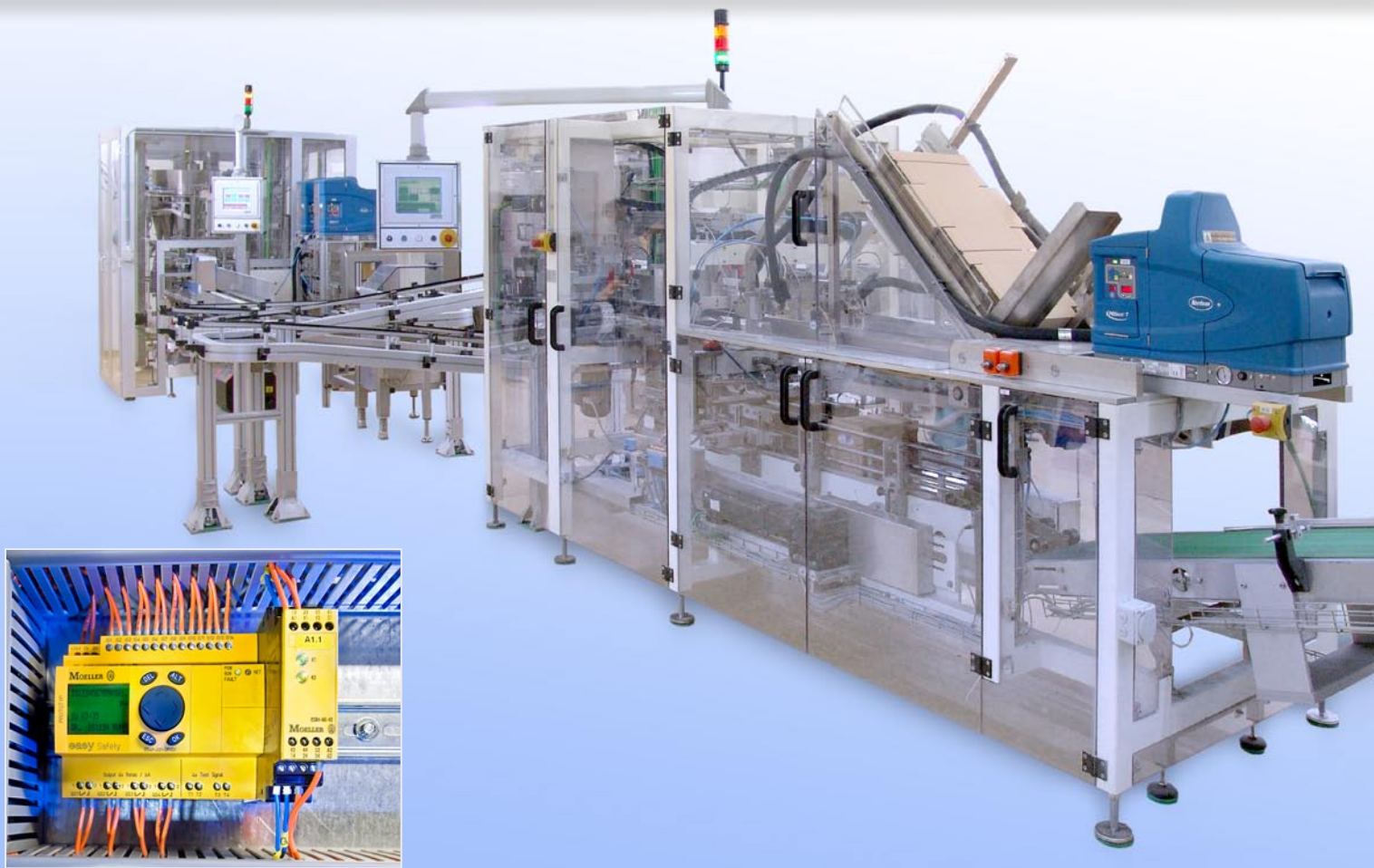
easySafety monitors all door and emergency-stop circuits, and communicates with the motor control system via Profibus DP.
