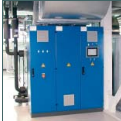
Control panels for heating, ventilation, air conditioning with integrated TFT touch panel operation
